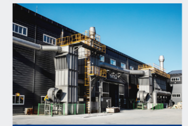
Dust Collecting System
